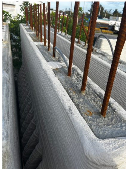
Figure 2D: 3D-printed component filled with interior core concrete fill and wire lifting hooks
